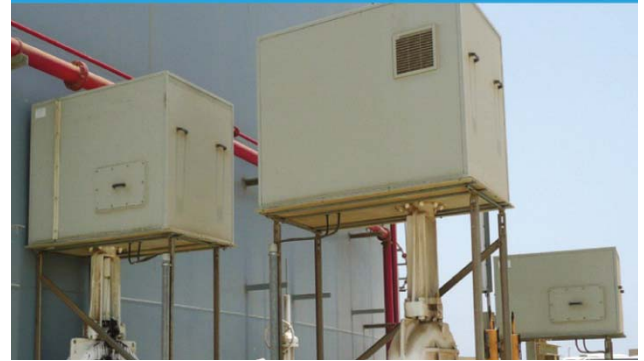
Fire Shelter for Valve- Actuator
